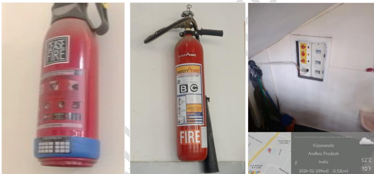
Plate 11: Fire extinguisher inside the campus and the server room
