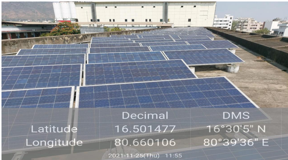
Solar panels on the rooftop of the main block
