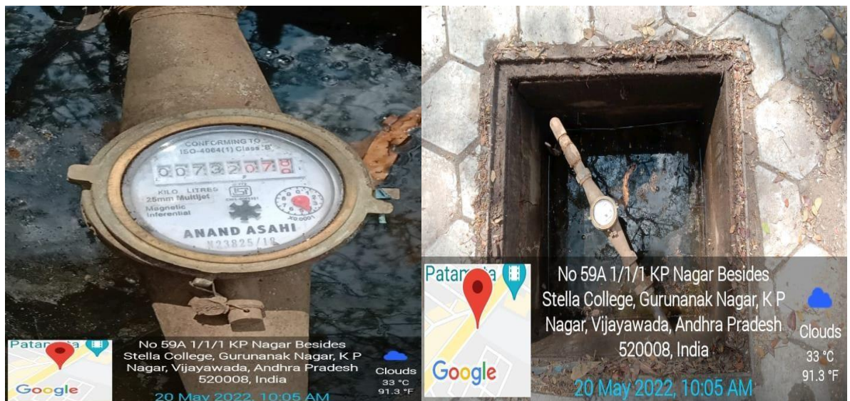
Water meters in the campus
