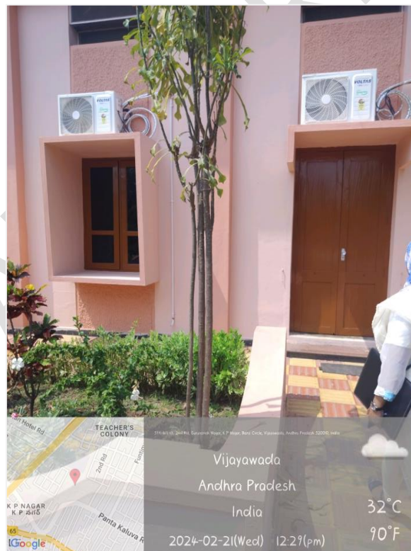
Plate 6: Outdoor units of the air conditioners in the campus
