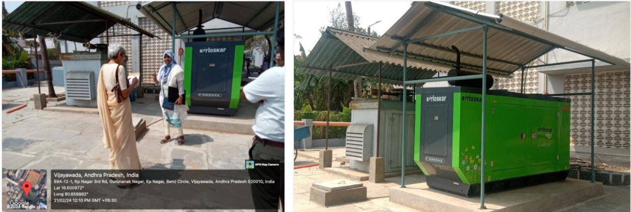
Plate 5: On-site transformer connected to all blocks
