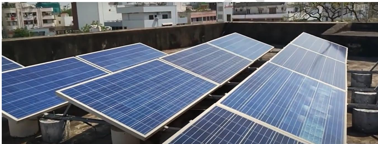
Plate 4: Rooftop solar panels in premises (Source: Institutes official media handle)
