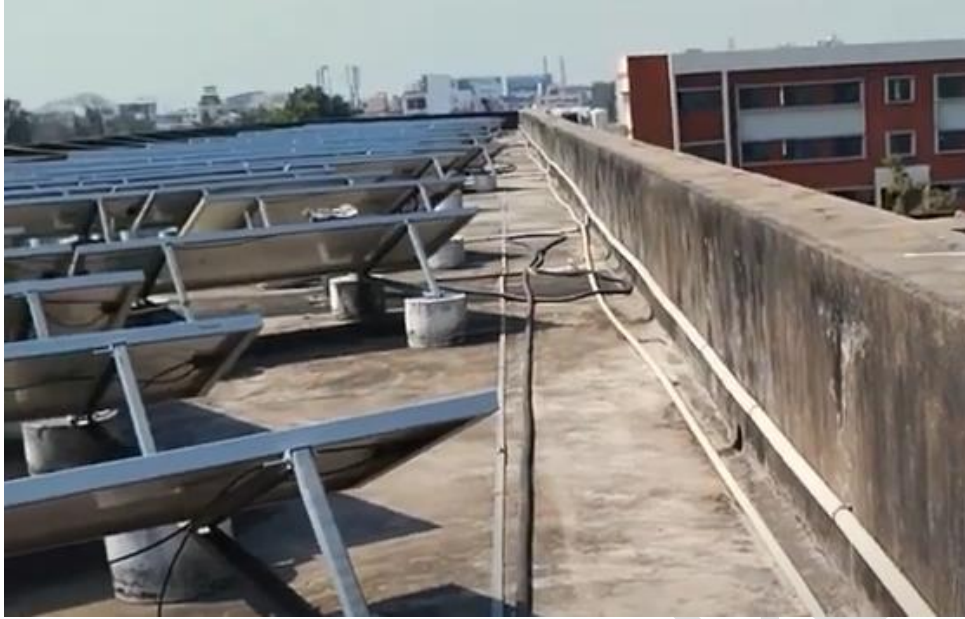
Plate 7: Solar panels on academic blocks rooftop (Source: Institutes official media handle)
