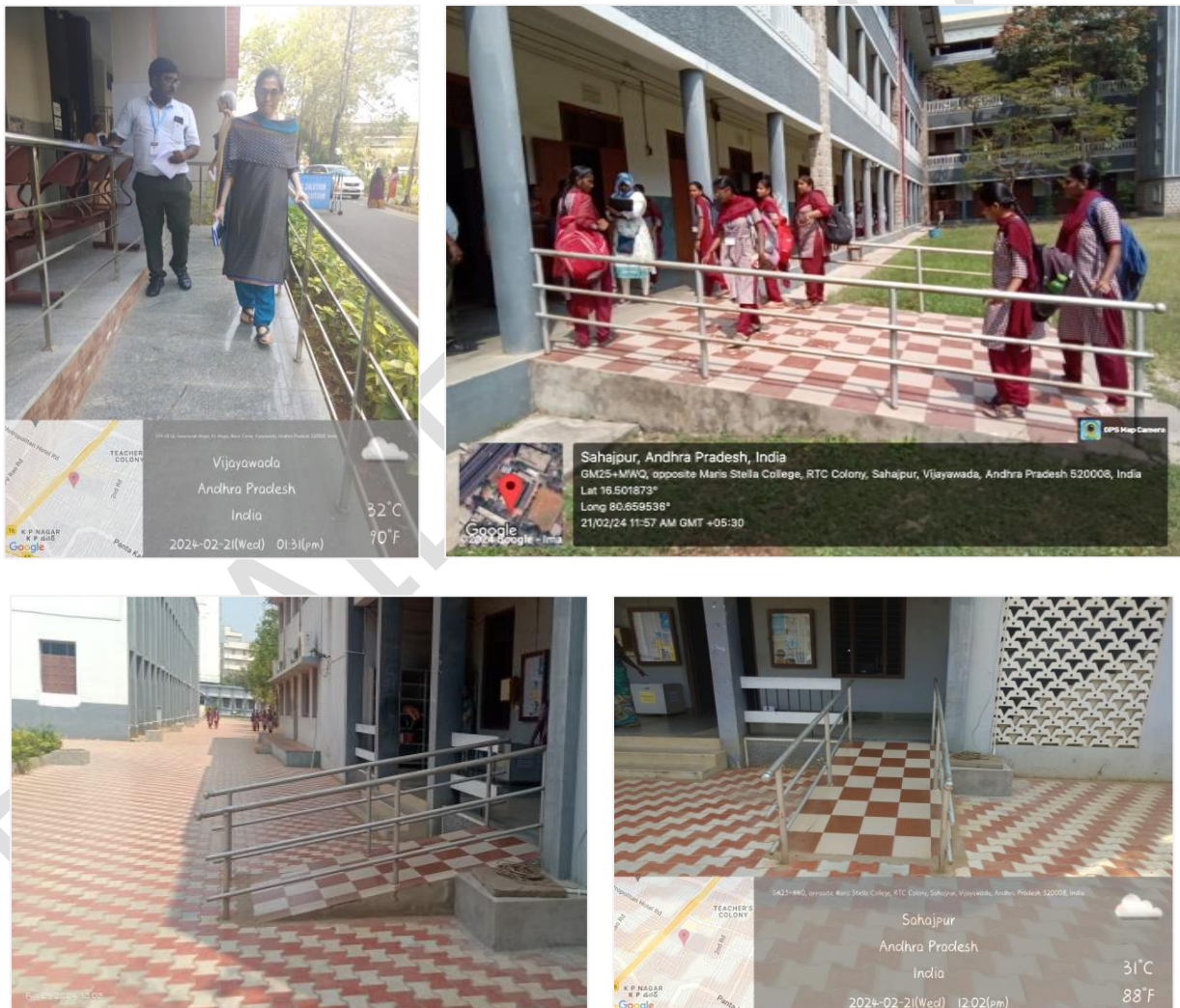
Plate 4: Ramps with handrails on both sides and non-slippery material, appropriate slope fair enough for wheelchair access without any inconvenience
