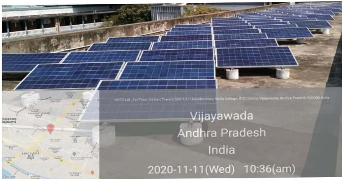
Solar panels on the rooftop of the main block
