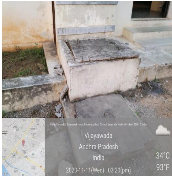
Rain water collection sump
