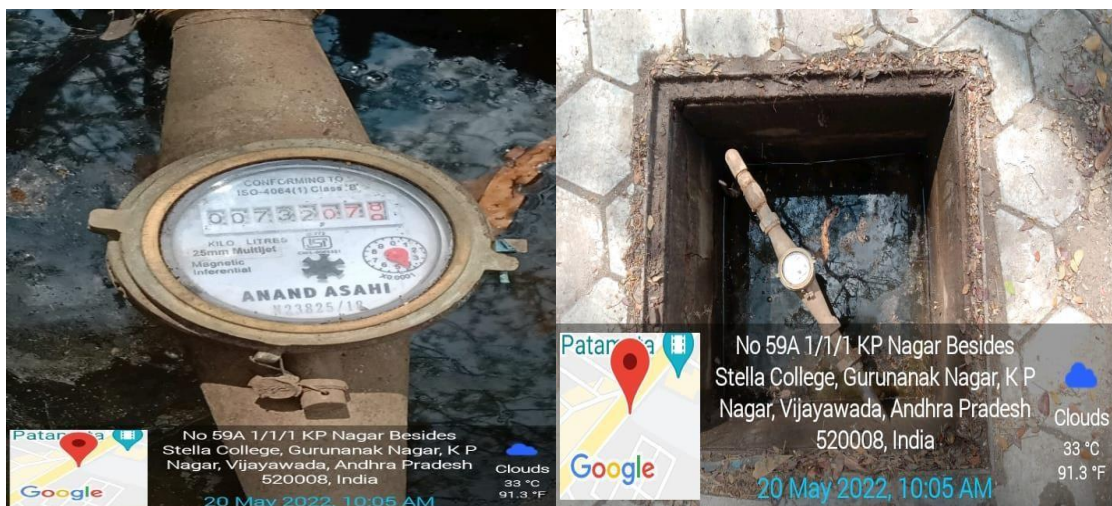
Water meters installed in the institution
